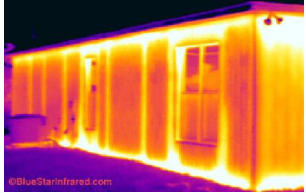
The exterior walls of this CBS type construction home are poorly insulated and wasting energy
